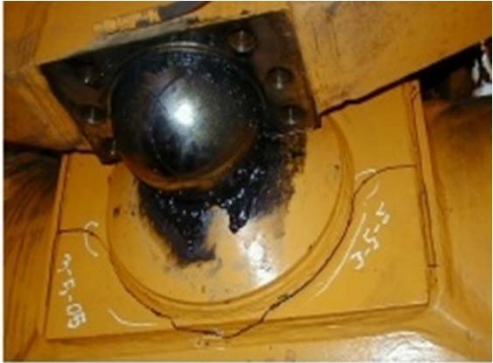
Cracked or broken Ball or Slab.
